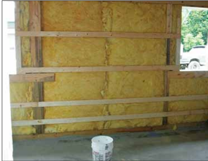
Figure 4. Fiberglass blanket insulation sandwiched between interior and exterior girts of a post-frame building
