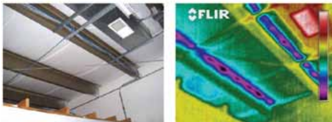
Figure 8. Thermogram shows similar temperature profiles for adjacent purlins.
