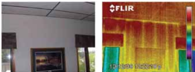
Figure 15. Thermogram shows lower surface temperatures in areas backed by wood studs.
