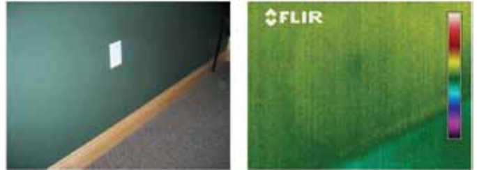
Figure 3. Thermogram indicates no abnormal heat transfer at the receptacle.
