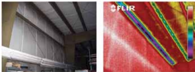
Figure 9. Image shows lowest temperatures occurring where insulation is compressed by eave strut. Exterior corners in all buildings are generally associated with greater heat loss per unit area.
