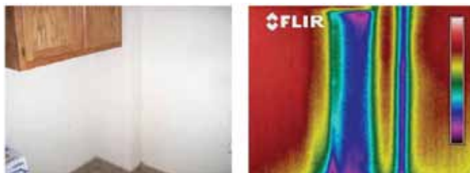
Figure 10. Covering around each steel column showed a similar temperature profile, a pattern indicating elevated heat transfer at column locations.
