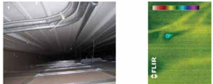
Figure 5. Cavity above suspended ceiling. Although no signs of air infiltration or exfiltration at panel seams appear, a spot on the electric conduit does register a colder temperature than that of the surroundings.
