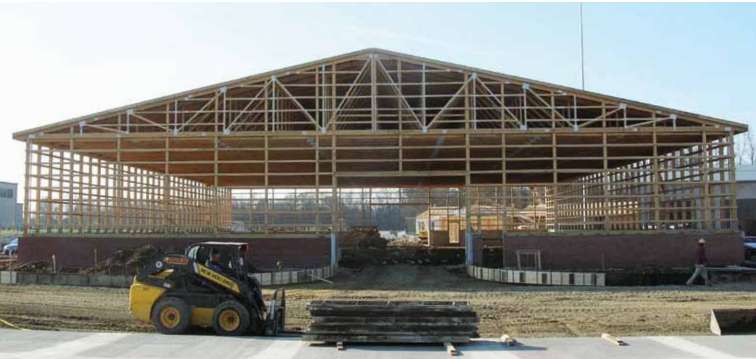
A 115-foot span truck storage building, shown here during construction was the first post-frame building finished in the ODOT project. It is located near Columbus. Photo courtesy of Jerome M. Scott Architects and Miller Watson Architects.
